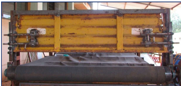
Fig. 4. FYM flow control gate
